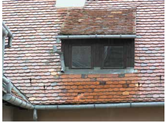
Fig. 6 Problems caused by lack of maintenance
