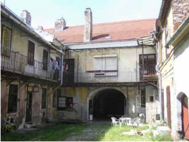
Fig. 5 Present run-down condition of the courtyard of an old town house
